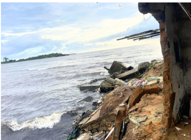
Effect of sea erosion on the Downtown beach in Greenville
